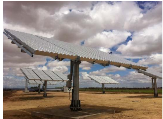
Fig. 6: CPV plant installed by BSQ with Daido modules in Villa de Don Fadrique (Toledo, Spain). Picture courtesy of BSQ.
